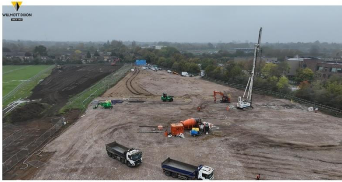
Image of construction vehicles working on stripping the site's topsoil and ground-cutting on Hopescourt School's permanent site in Walton-upon-Thames
