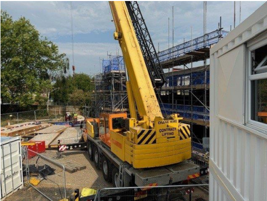
Image of the crane in position lifting the prefabricated roof panels from the ground to the roof at Fordway Centre in Ashford.
